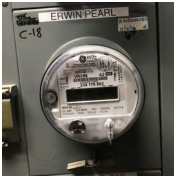
TERMINAL 3 CONCOURSE HK APEX ELECTRICAL METER
