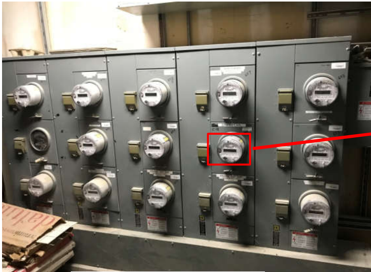
ELECTRICAL METER PANEL - TERMINAL 3 CONCOURSE HK APEX PENTHOUSE LEVEL
